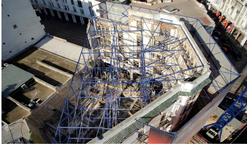
Figure 4: Example of Façadism: Building of the General Society in Casablanca Shoring Works, Photo Taken by Ibtissam Kourdou. 2013.
